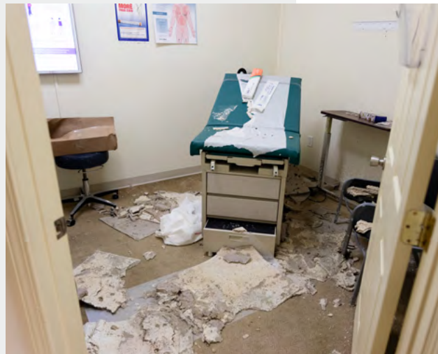
Avicenna Free Clinic in Panama City, Florida, suffered major damage from Hurricane Michael in 2018. Photo used with permission from Avicenna Free Clinic.
