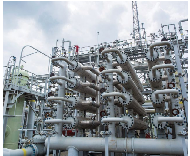
Grissik Gas Plant, South Sumatra
