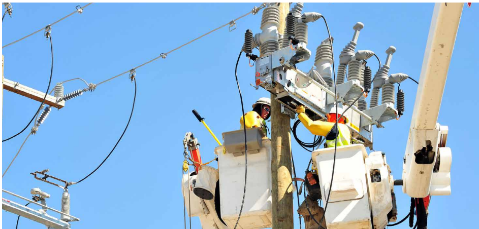
Data centers and warehousing are examples of business growth that is driving investment in new substations and distribution equipment in our service areas.
